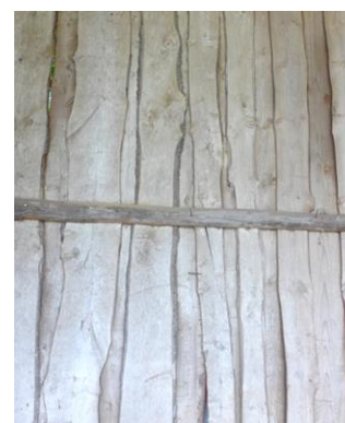
Fig. 4: inside of boards on boards on a barn, Västra Götaland. Photo by R. Carlsson.
