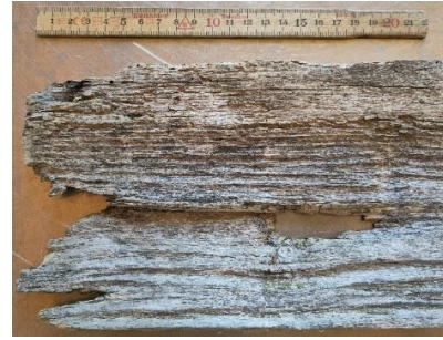
Fig. 2 : A "tavillon" of Alder from the façade on Fig. 1 is showing a nail hole, which has become bigger and where crack formed from it to the edge.
